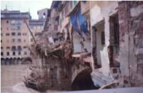
Damage at Ponte Vecchio
